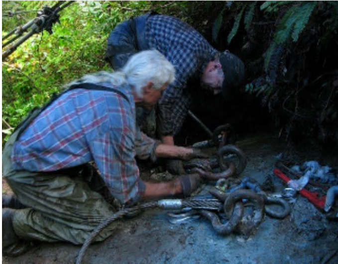
Kel and Bob install new anchor pins on the Gayle McGee bridge.
