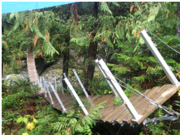
Gayle McGee Bridge before repairs
